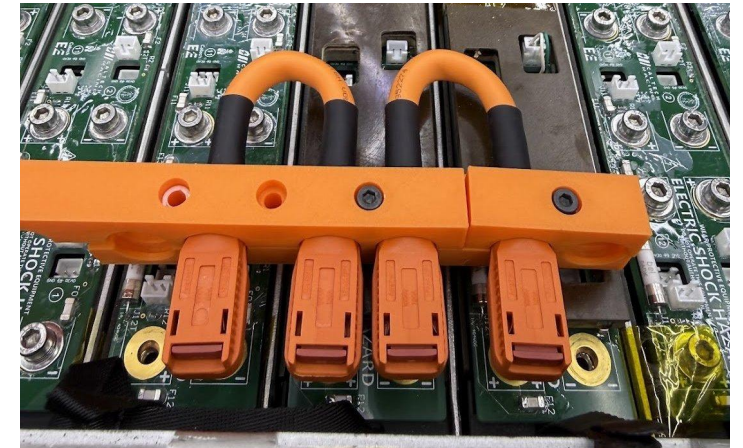
4 · Printed separators on the battery plugs
